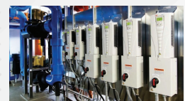
► VFD Pumps & Cooling Towers
